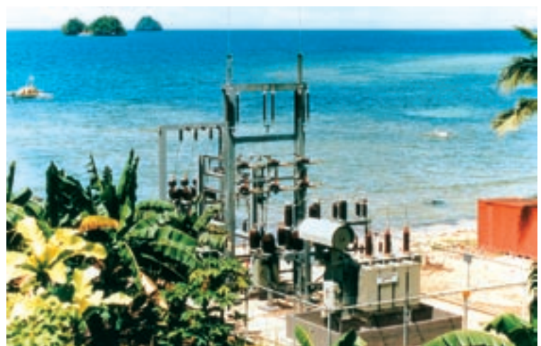
34.5 kV shore substation submarine cable project Mindanao, Philippines
